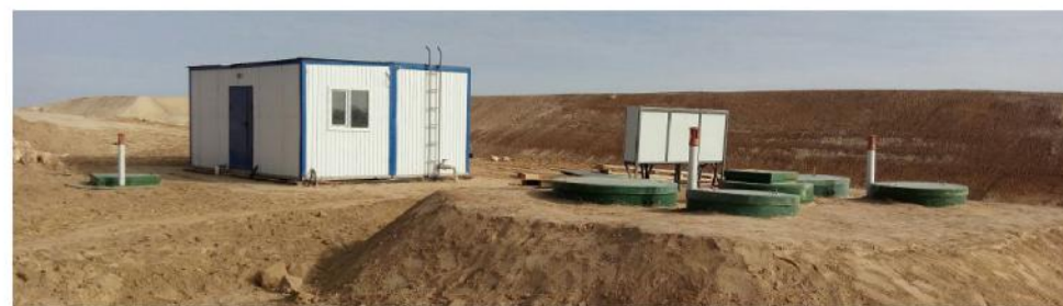
Waste water treatment system at Kyruk Port, Mangystau region
